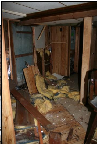
Building is not ADA compliant (handicapped accessible) and serious mold and water damage conditions exist throughout the basement
